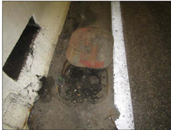
Figure 218: Typical debris around the hydrant
