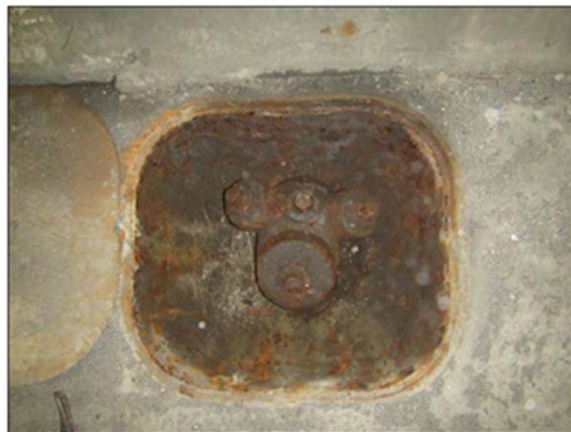
Figure 219: Typical corrosion of the hydrants
